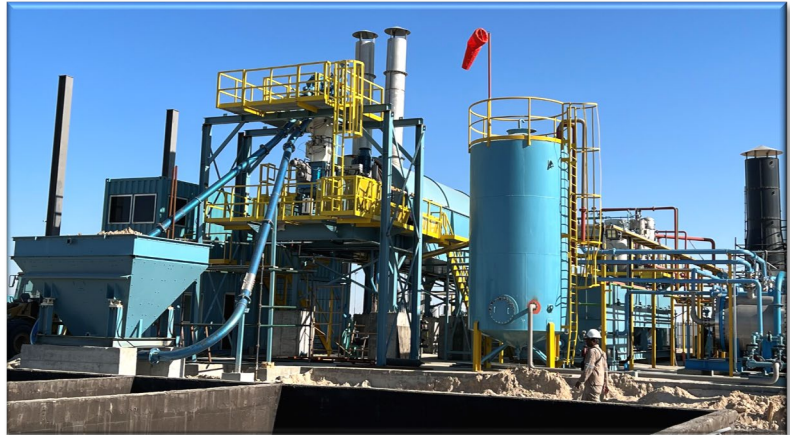
Kuwait Indirect Fired Thermal Desorption Unit
